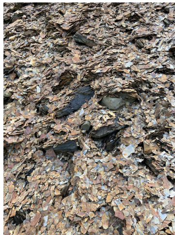
Figure 2. Exposed Sunbury Shale on KY-32 at bridge over North Fork of Triplett Creek.
